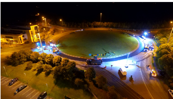
Night time surface restoration works at Drumlonagher roundabout, Donegal Town to minimise traffic disruption.
